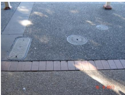
Photos courtesy of Essential Energy
