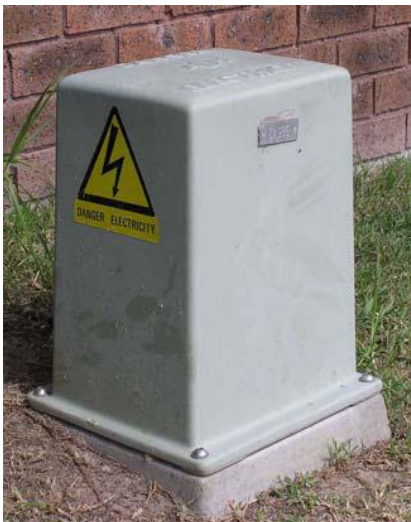
Photo courtesy of Ausgrid
