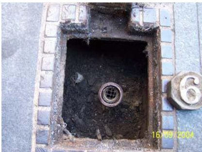
Access cover opened – the 6 on the cap indicates the number of CO 2 cylinders to be injected
