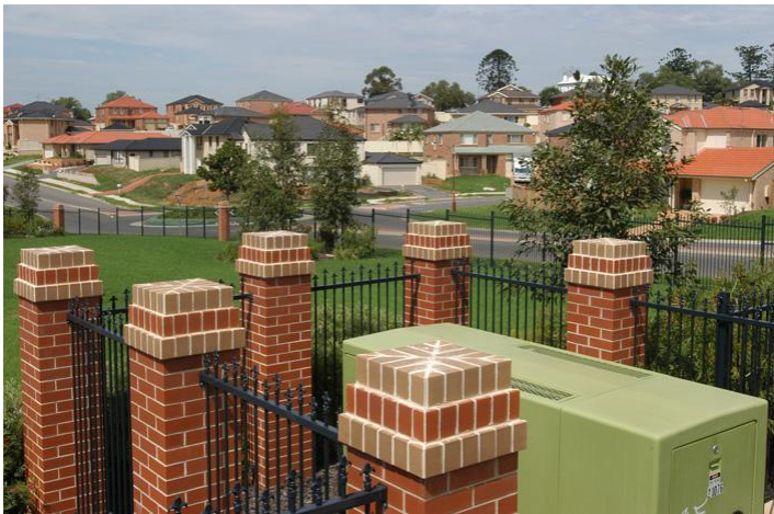
Kiosk substation in new housing area
