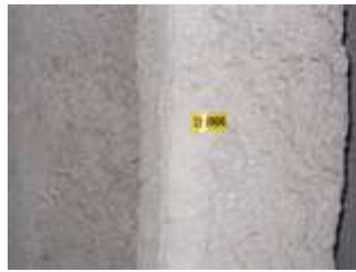
Sprayed limped asbestos to steel column
