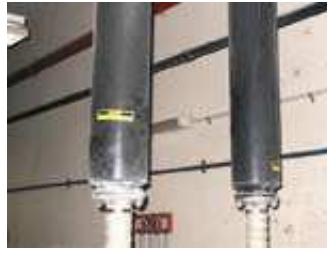
Asbestos lagging inside steel; Asbestos vinyl tiles lining to pipework
