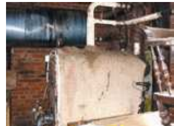
Asbestos insulation (friable) as lagging to boiler and pipes
