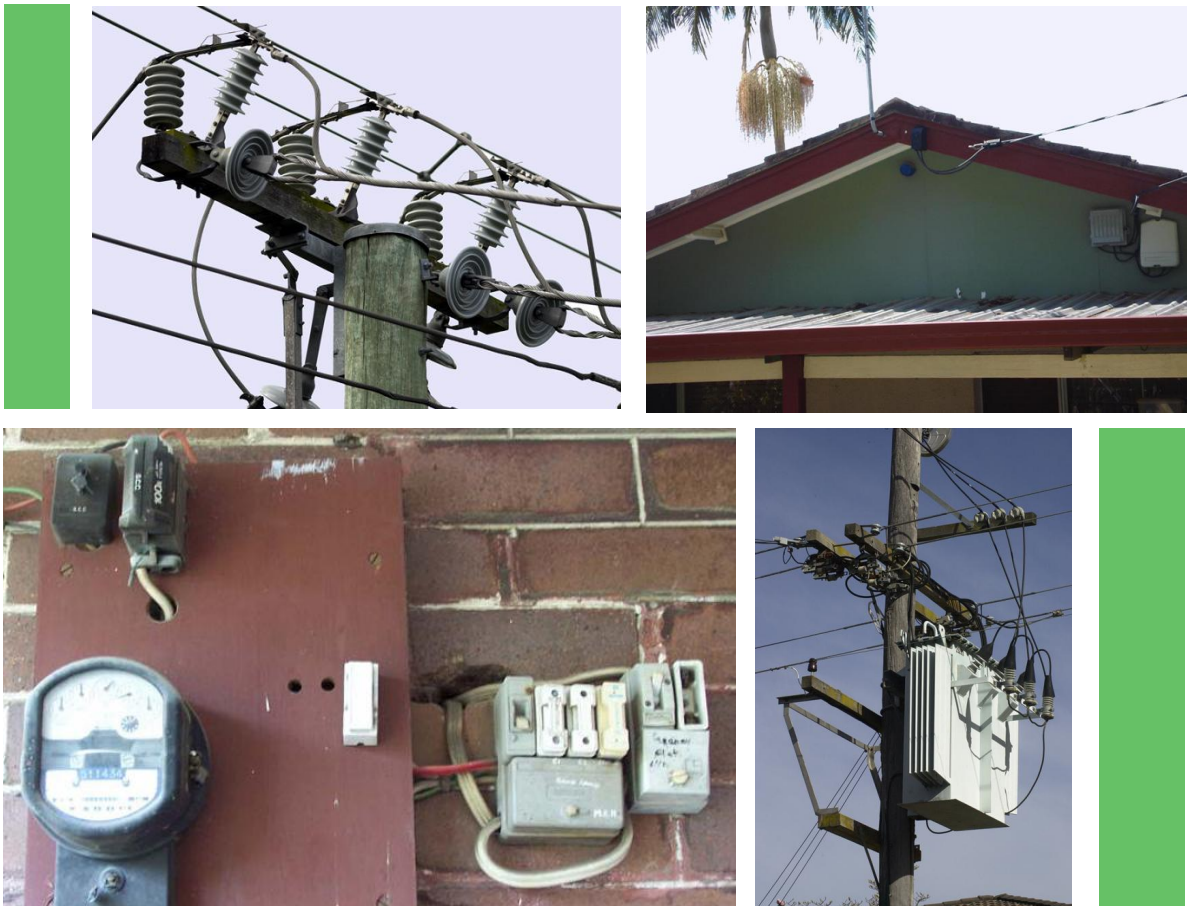
Top left, top right, bottom right photos courtesy of Endeavour Energy
