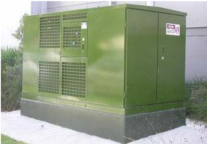
Kiosk (or padmount) substation
