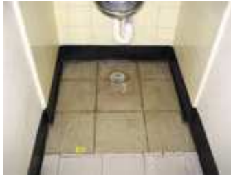
Asbestos vinyl tiles
