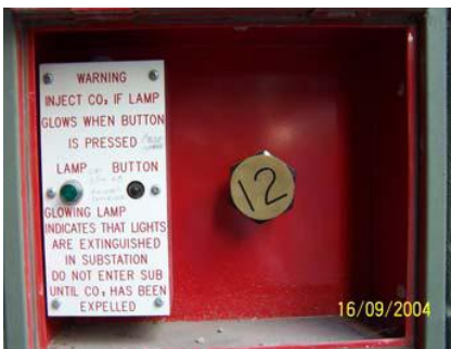
Wall box opened – 12 indicates the number of CO 2 cylinders to be injected
