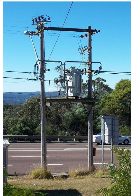
Double pole-mounted substation
