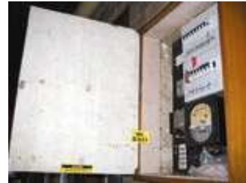
Zelemite meter board in asbestos-fibre-cement-lined meter box
