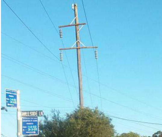
Photo courtesy of Ausgrid
