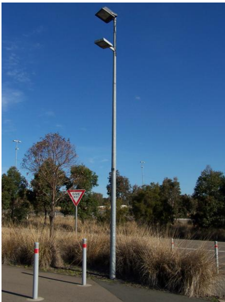
Street light columns
