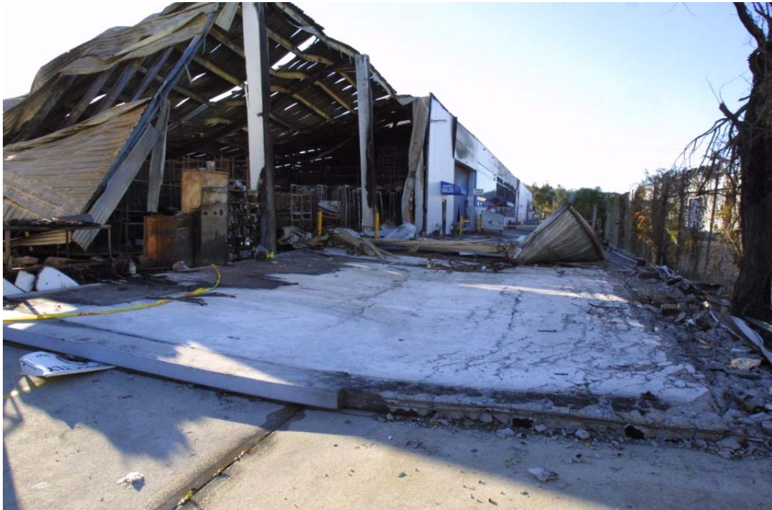
Figure 2. A fallen wall panel
