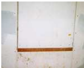
Asbestos fibre cement wall panel to riser
