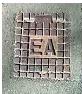
Ground level access box for CO 2 injection – showing Sydney County Council (SCC) and EnergyAustralia (EA) markings
