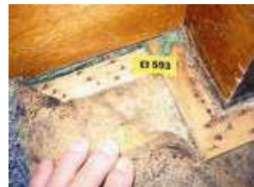
Asbestos vinyl tiling under carpet
