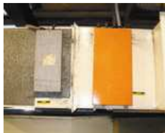
Internal millboard (asbestos) lining to inline duct heaters
