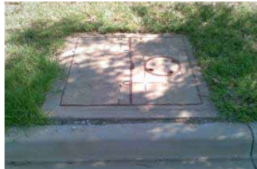
Figure 1 - Large hydrant cover
