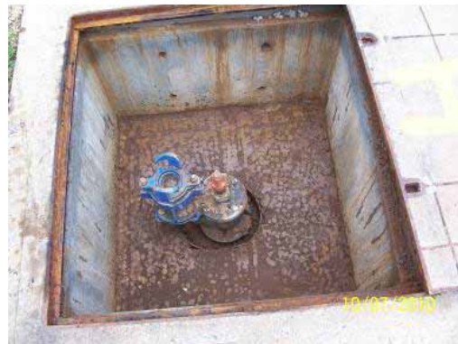
Figure 2 - Pit containing hydrant and isolating valve
