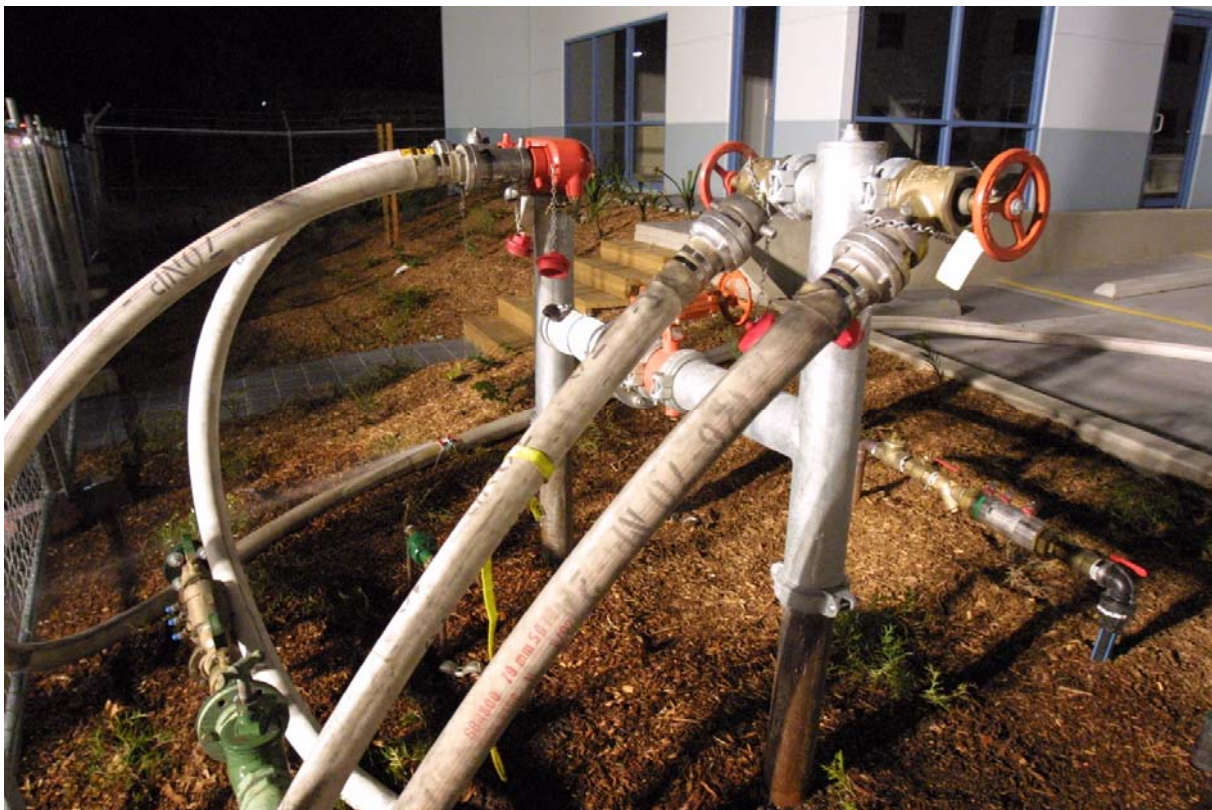
Figure 1 AS 2419 hydrant booster system
