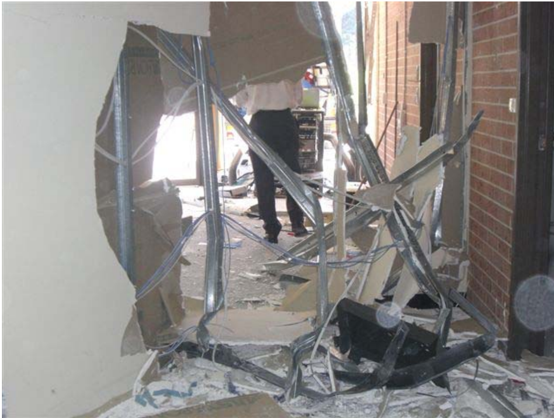
Figure 6 Internal partition wall 20 metres from the ATM destroyed when the back was blown off the ATM by the explosion shown in Figure 4
