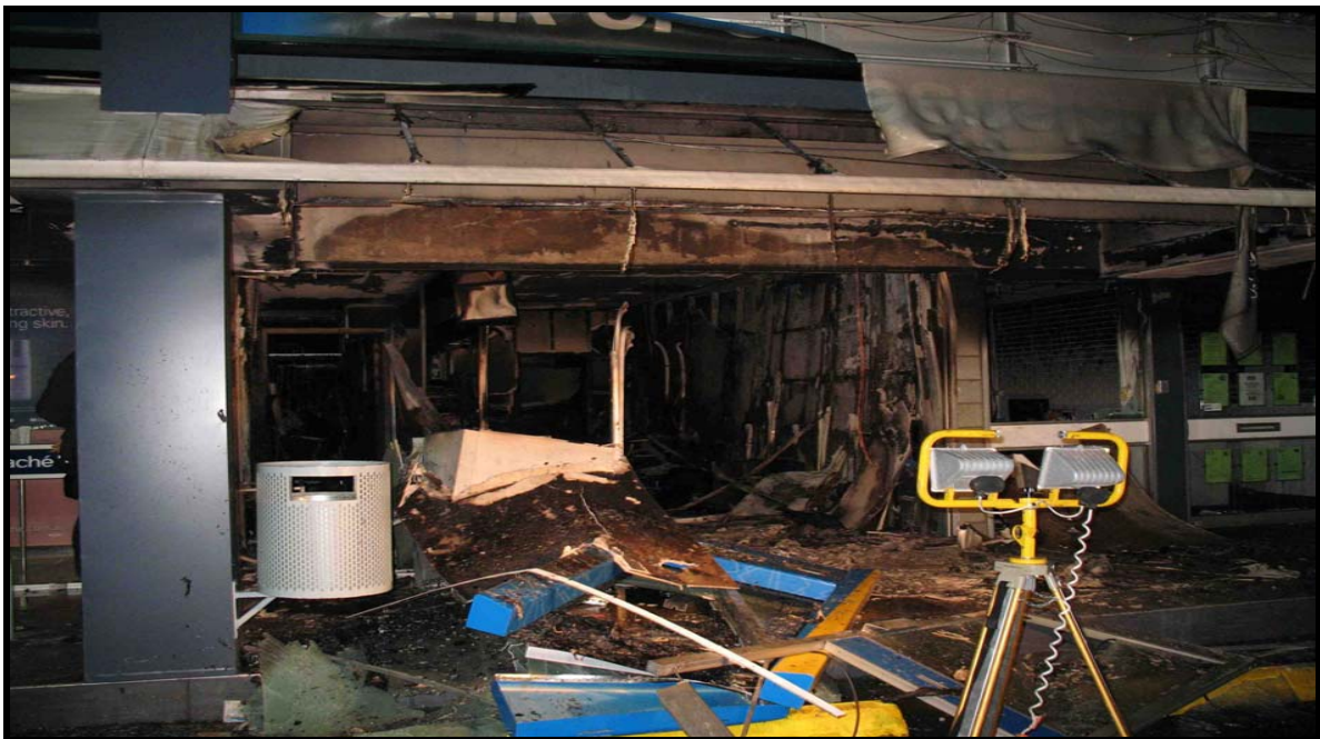
Figure 3 Shop front destroyed and awning damaged by force of explosion
